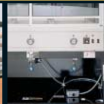
Hot Deli temperature controls and drains
